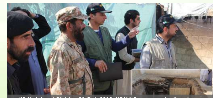
KP Malakand Division 31 Oct, 2015: NDMA Teams conducting damage assessment for compensation verification process at village Killa Pata, U.C Malanjaba, Tehsil Charbagh, District Swat.
